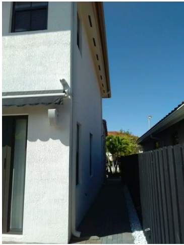
All Exterior Openings Are Impact Rated
