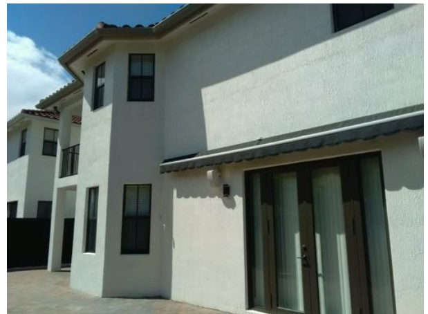
All Exterior Openings Are Impact Rated
